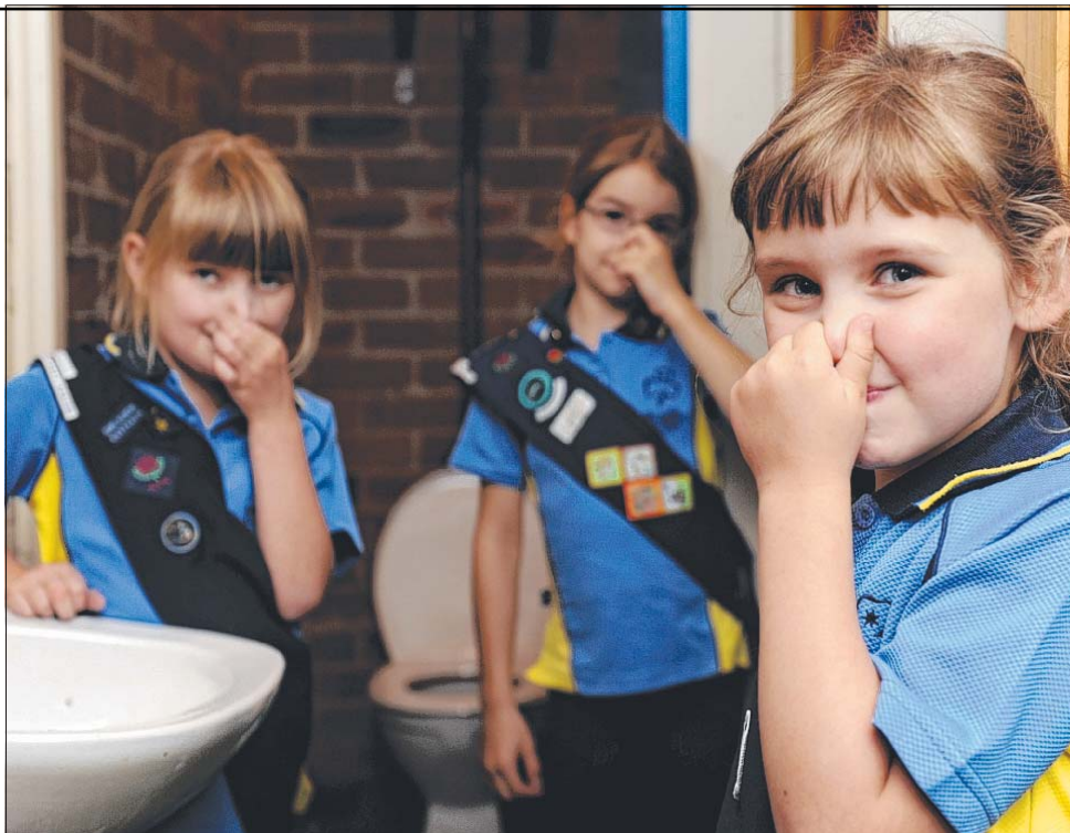
Elanora Girl Guides Kayley Dixon (front), with Sophia Lauber and Ruby Warde, would like to get their toilets fixed up, as they smell and even the lights don't work.
